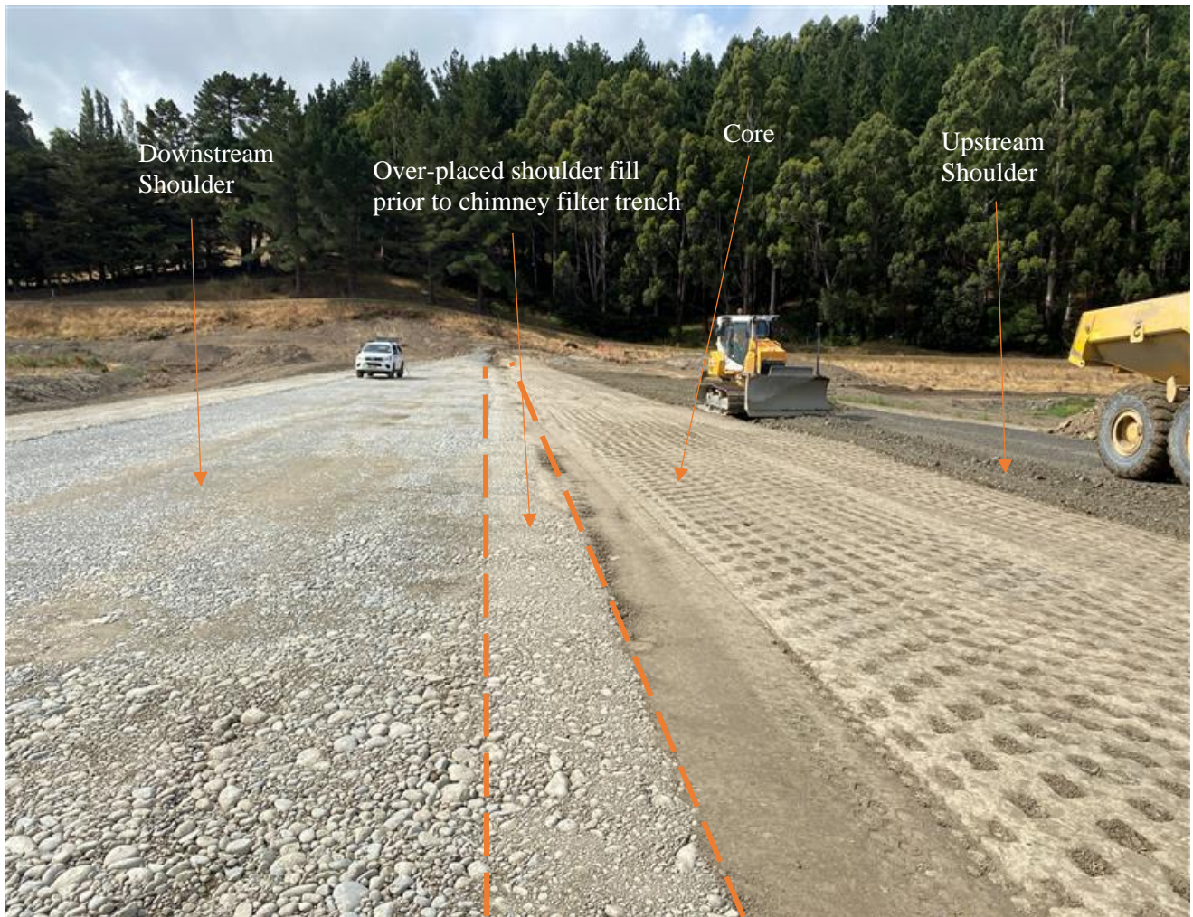
Figure 11. Placement of core and shoulder fills prior to trenching back to place filter fills.
