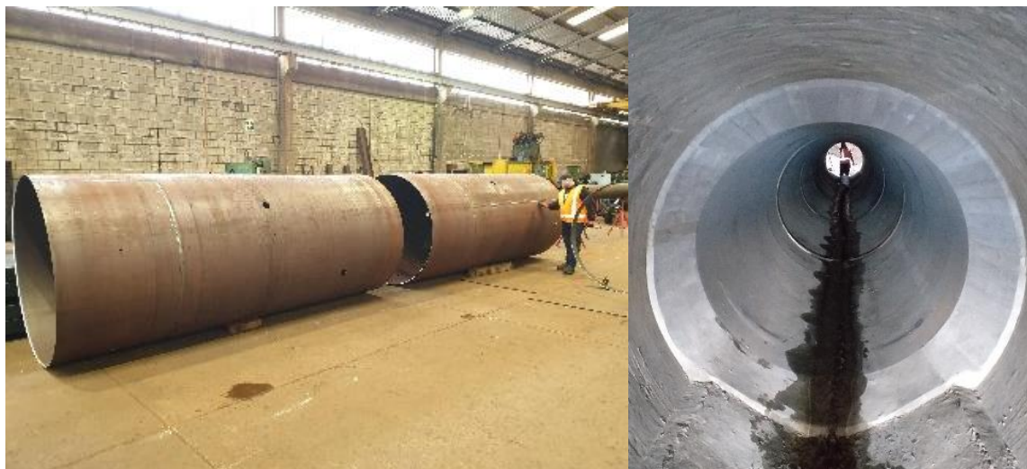
Figure 4: The SH35 culvert: steel liner sections on the left and post install on the right.
