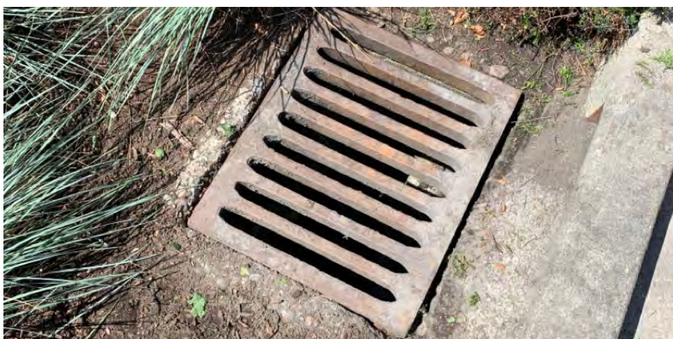
Moderate damage to concrete around CB, could be sign of water leakage. Condition score: 3
