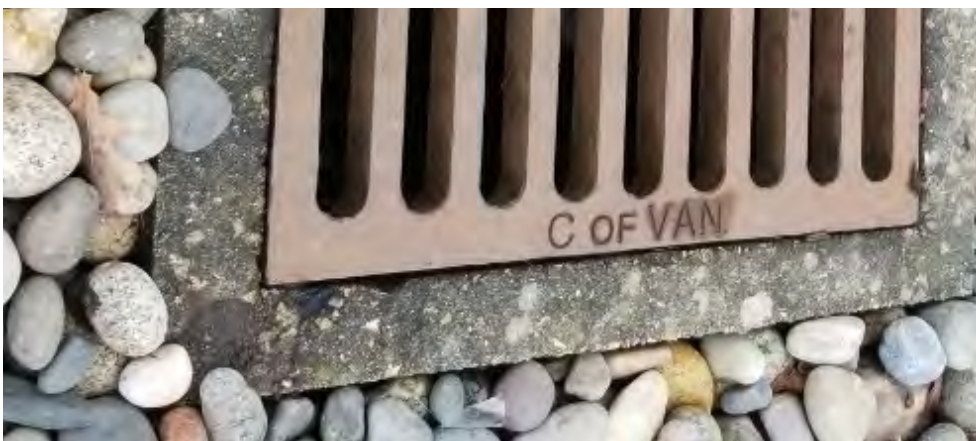
CB with minimal spalling on exterior Condition score: 2
