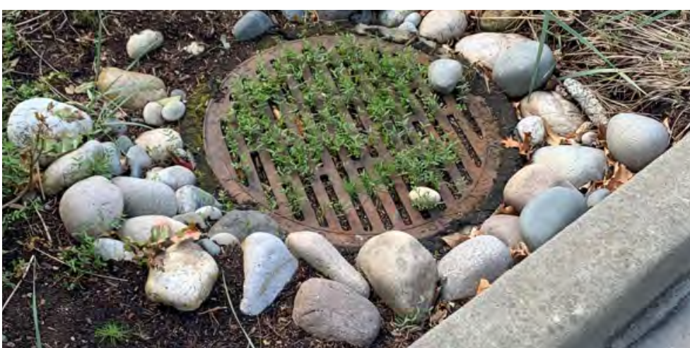
CB is filled with debris and non-functional. Could cause backups that create community risk. Condition score: 5
