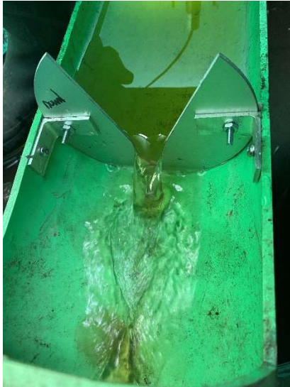
Photo 2-2: 45-degree V-notch Weir Installed to Facilitate Level Logging in the Underdrain of Bioswale #2
