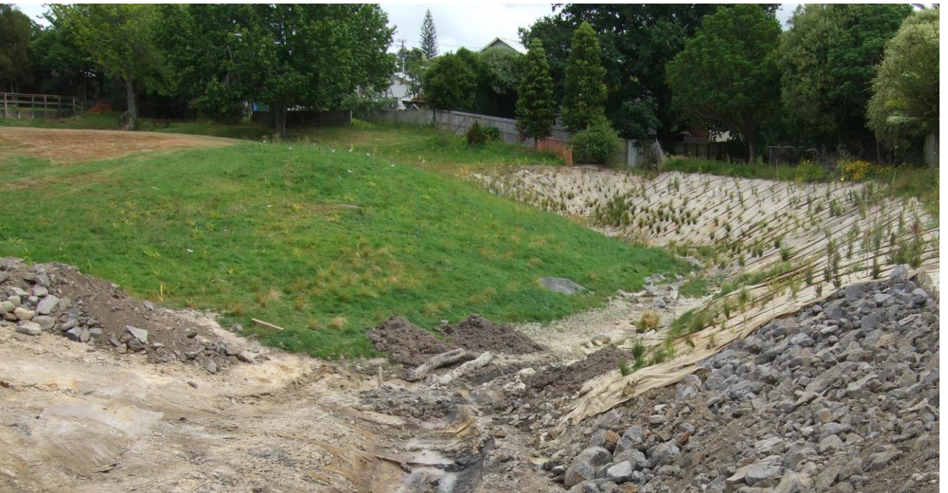
Photograph 4: Riparian planting and construction of habitat features for main channel completed. Levelling and sowing of grass on raised field complete.
