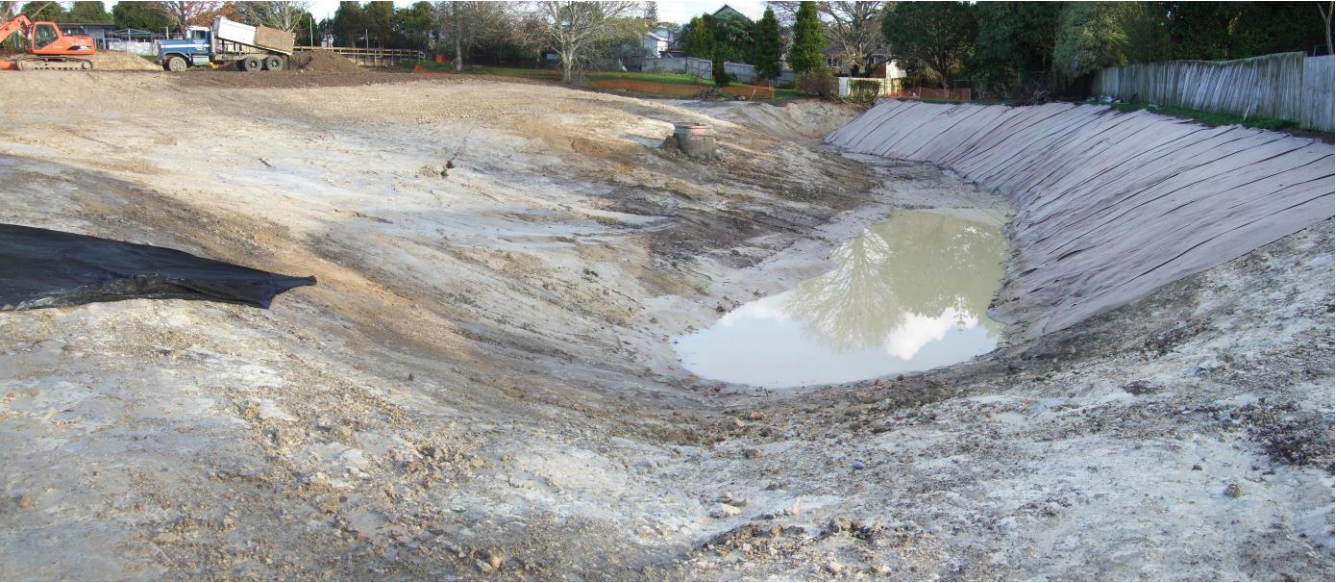
Photograph 3: The main channel excavated and sculpted to a natural contour. The fish passage feature yet to be constructed will be in the in foreground
