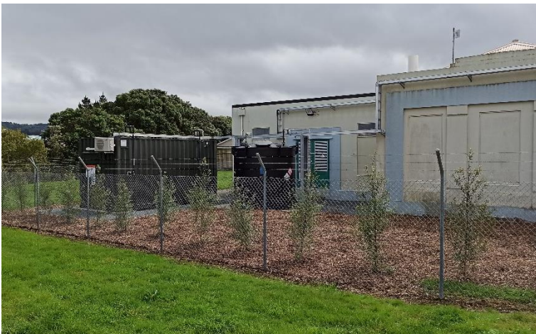
Figure 5: Gear Island WTP Fluoridation System
