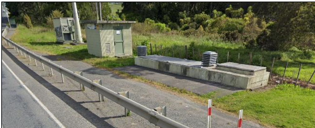
Figure 3: East Coast boost pump station within road corridor (4)
