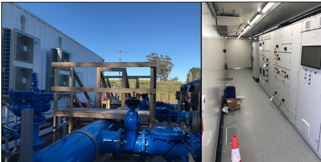
Figure 12: Prefabricated switchroom placed at the site
