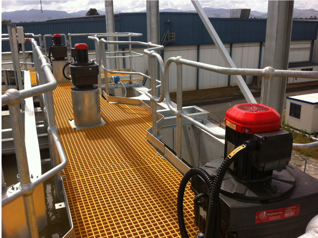
Photograph 2 – Flocculation Tank Mixers
