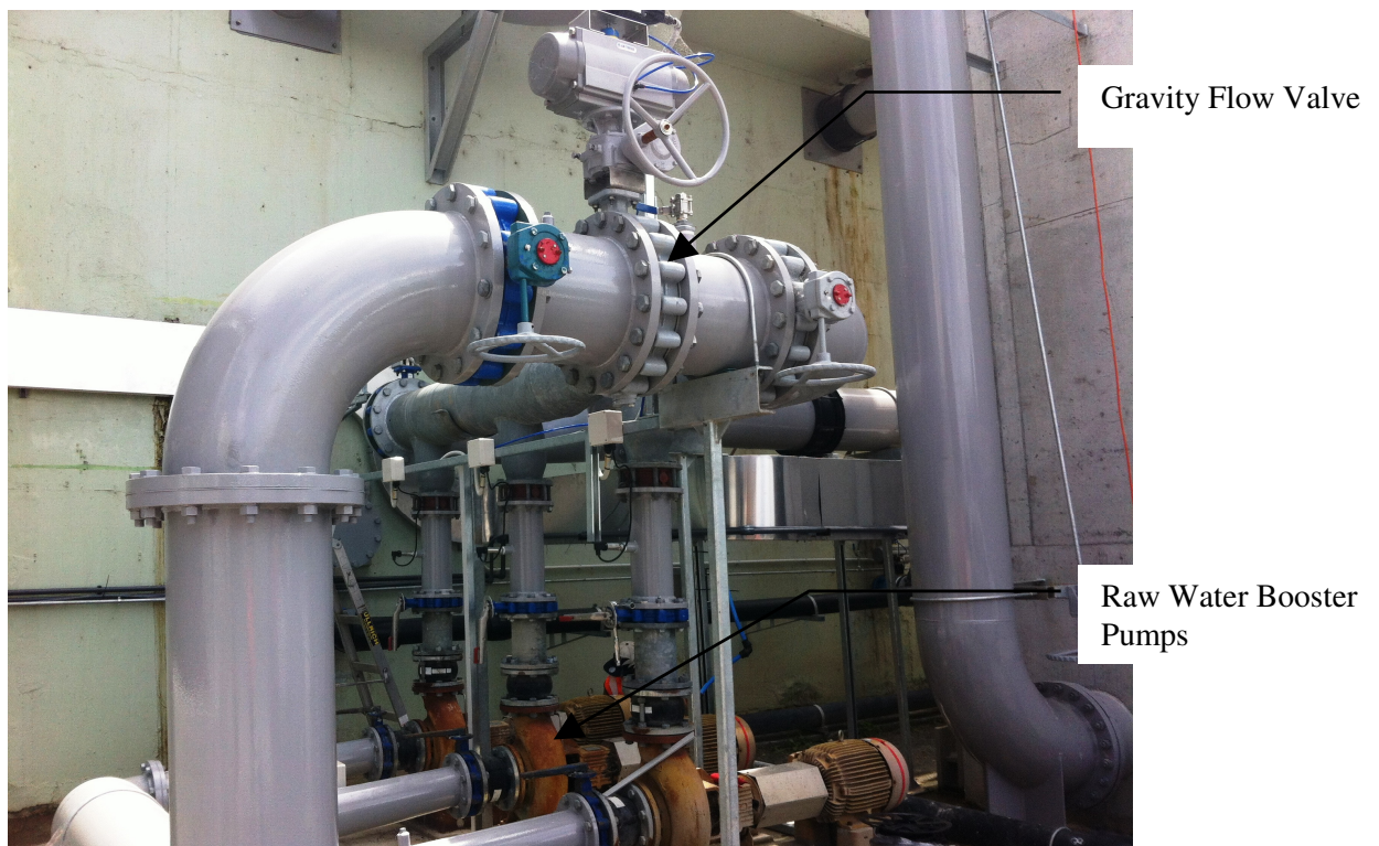
Photograph 1 – Raw Water Booster Pumps and Gravity Flow Valve
