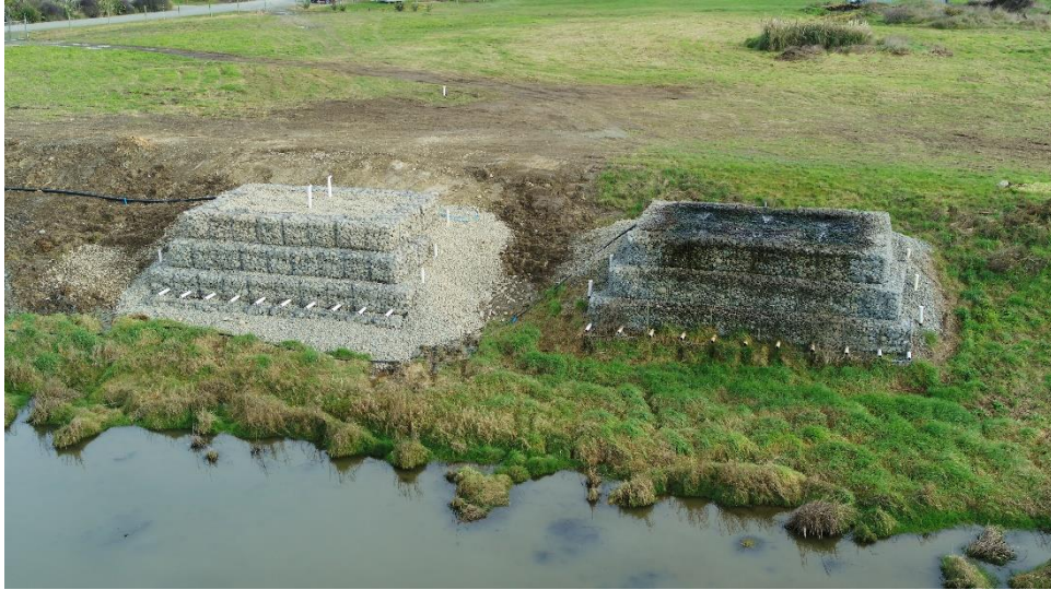
Photograph 1: Drone photo of the trickling filters following the recent completion of NTF number 2 (on left).
