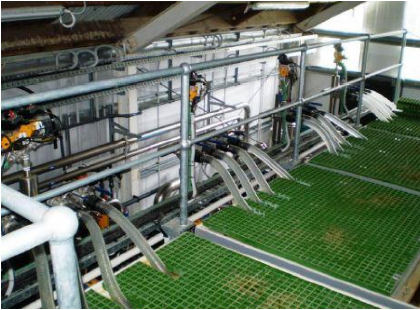
Photograph 3: Waikouaiti WTP membrane trains
