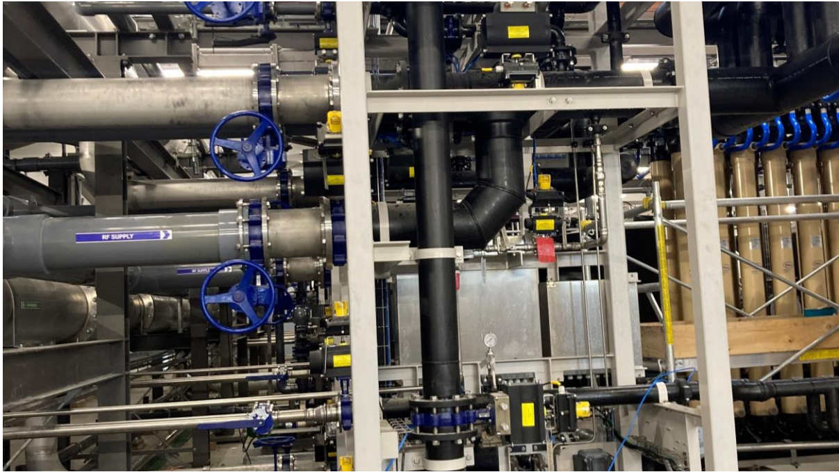
Photograph 3: Double isolation of pressure systems
