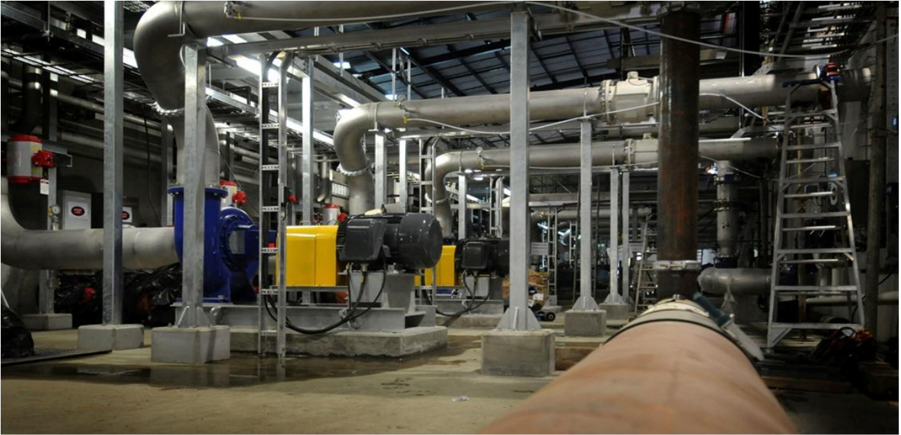
Photograph 4: Temporary Membrane Permeate to Waste Pipe Spool
