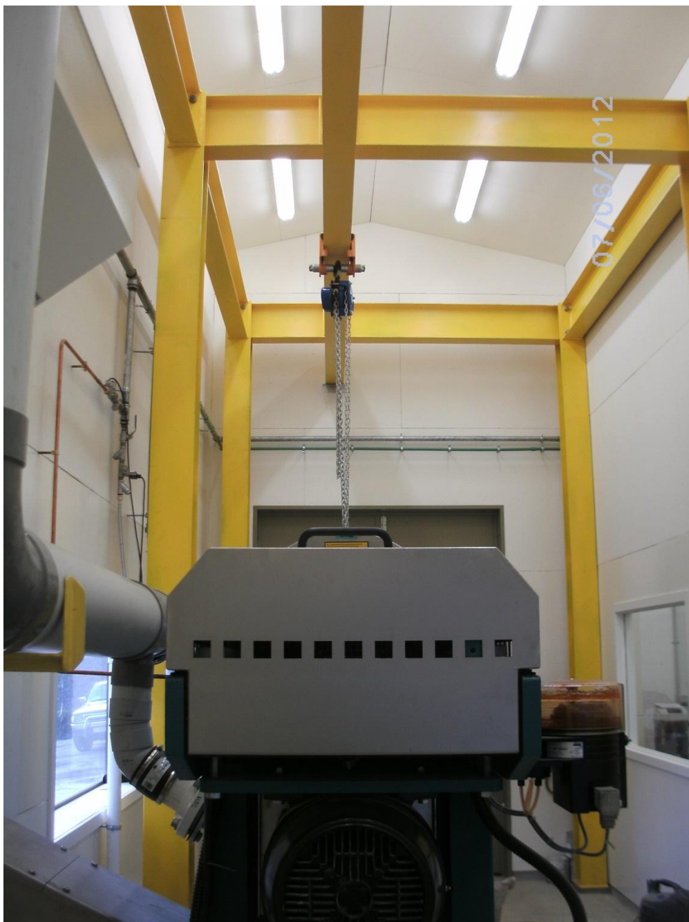
Photograph 5: Centrifuge UCD 305-00-32 and Gantry
