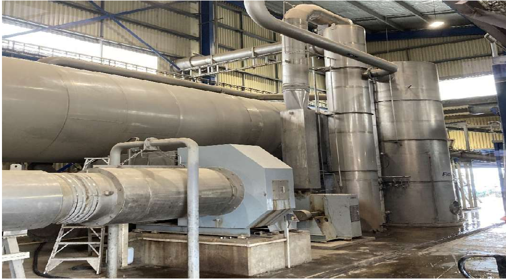
Figure 7: Sludge drying facility at Seaview wastewater treatment plant
