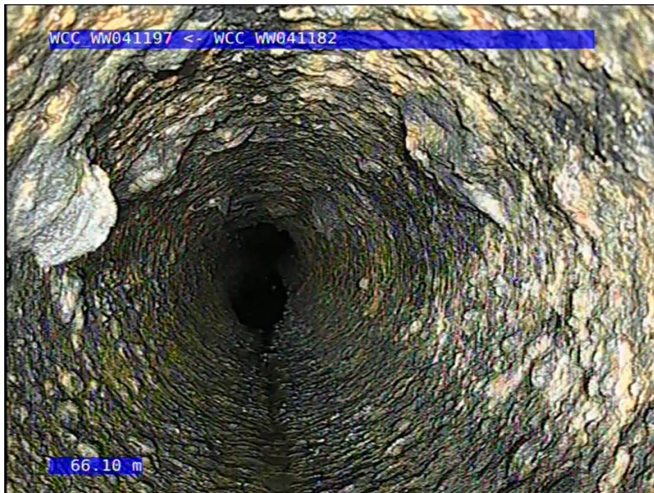
Figure 3: Internal condition of the existing cast-iron Featherston Street rising main prior to cleaning.
