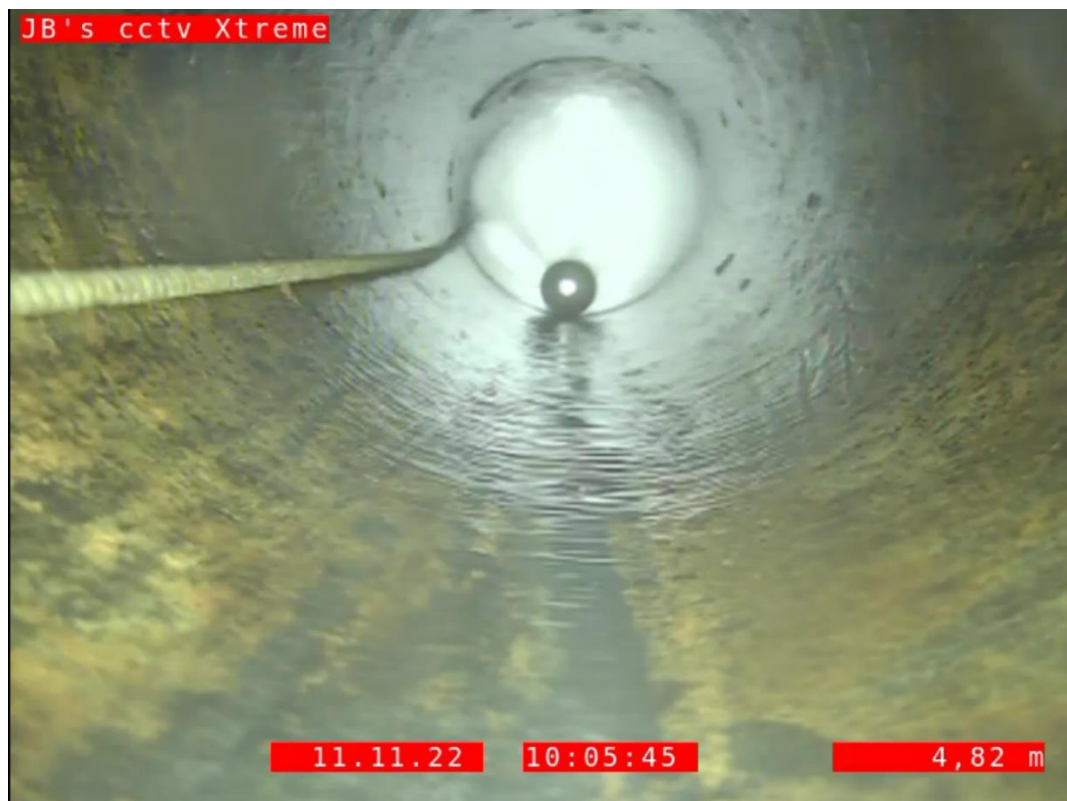
Figure 6: Internal condition of the existing cast-iron Featherston Street rising main after being flushed clean by a high-pressure jet (CH 4.82m).
