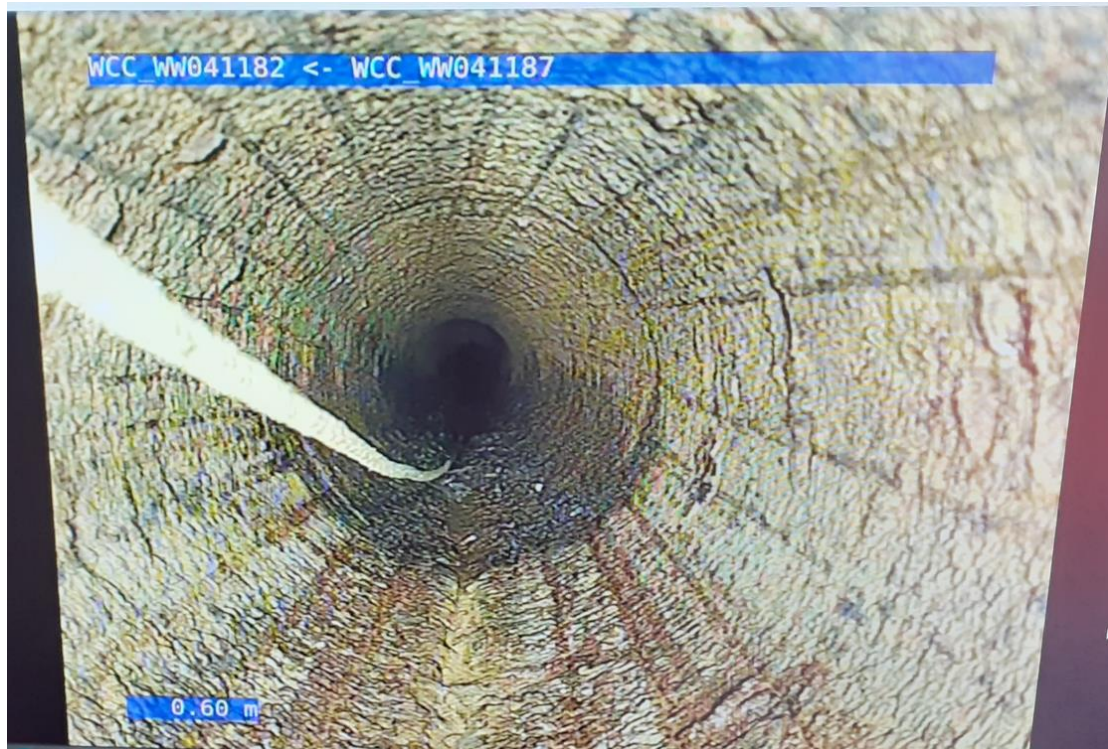
Figure 5: Internal condition of the existing cast-iron Featherston Street rising main after two passes of the mechanical scraper.
