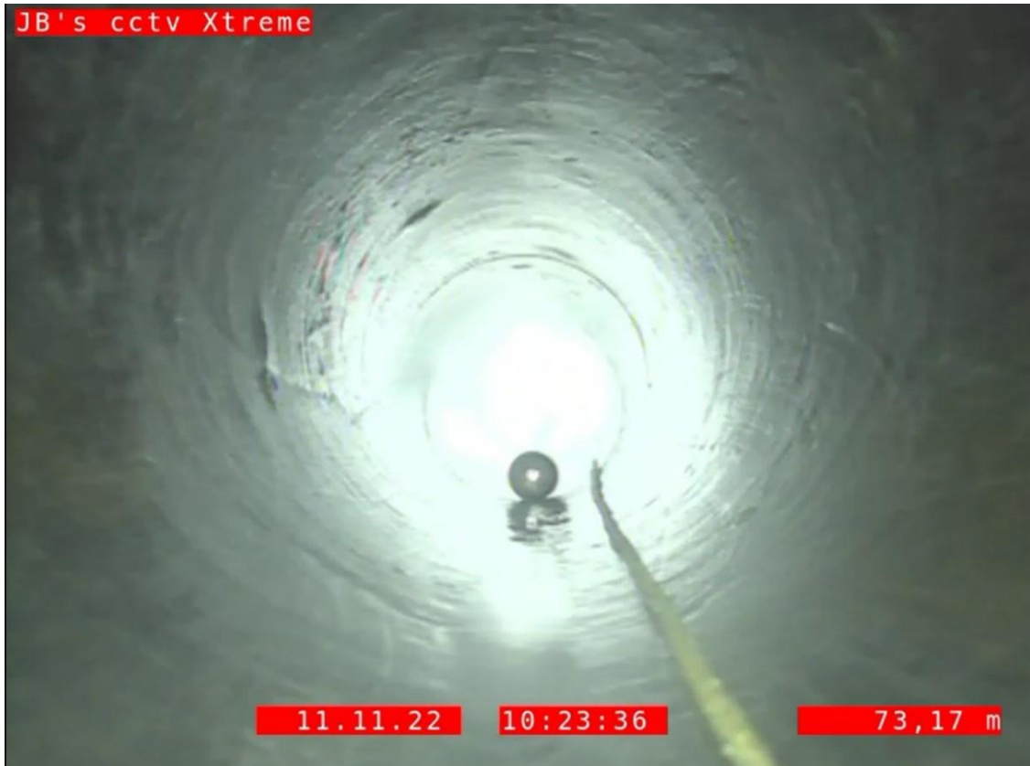
Figure 7: Internal condition of the existing cast-iron Featherston Street rising main after being flushed clean by a high-pressure jet (CH 73.17m).
