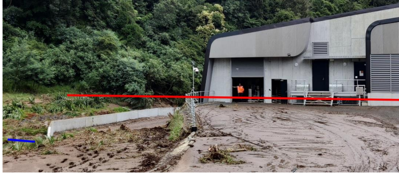
Photograph 7: Jan 2023 flood level.
