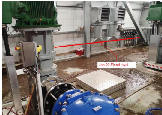
Photograph 8: Height of flood within the pump room.
