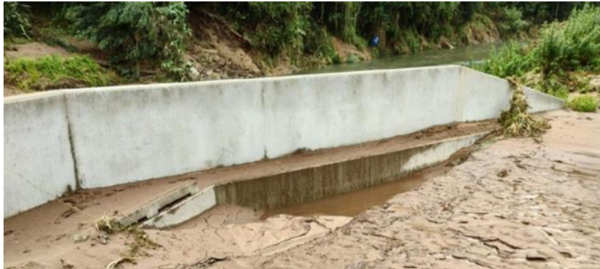
Photograph 15: Scour damage on downstream face of parapet wall.
