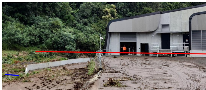
Photograph 1: post-flood photo showing indicative typical stream level (blue) and flood level (red)
