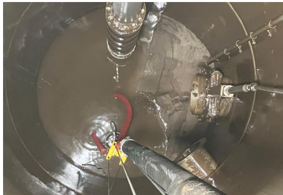
Photograph 14: Silt build-up in wet well.
