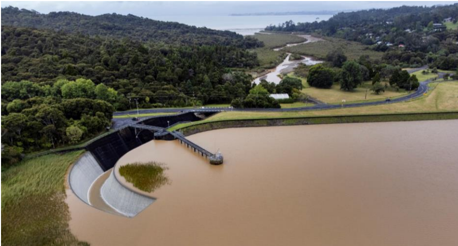
Image 2: Lower Nihotupu Dam in the Waitākere Ranges was affected by slips, causing the level of turbidity to rise.
