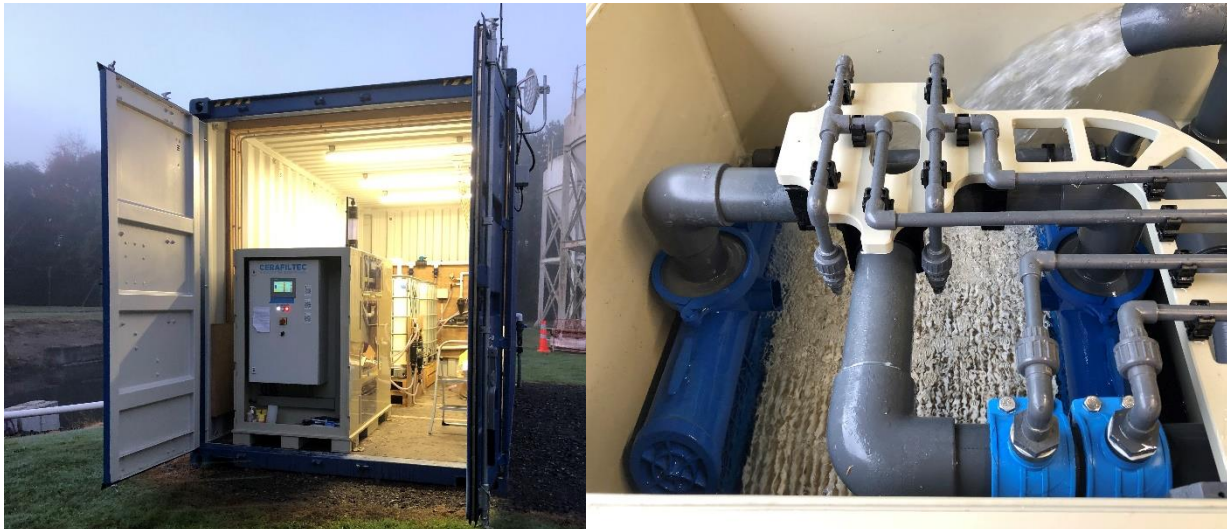
Figure 2: Top left: the pilot plant container with the Cerafiltec membrane skid visible in the front. Top right: View of the filtration tank while raw water enters. White membrane sheets visible at the bottom. The small diameter lines are used for chemical cleaning, either spraying onto the membranes (CapClean), or injecting into the filtration/backwash line (CEB). Bottom left: 3D model of skid (from Cerafiltec). Bottom right: top view of skid with labelled components (from Cerafiltec).
