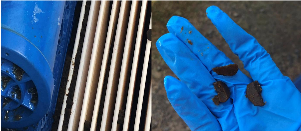
Figure 8: A misconfiguration resulted in sludging of the ceramic membranes around the 20th February 2023.
