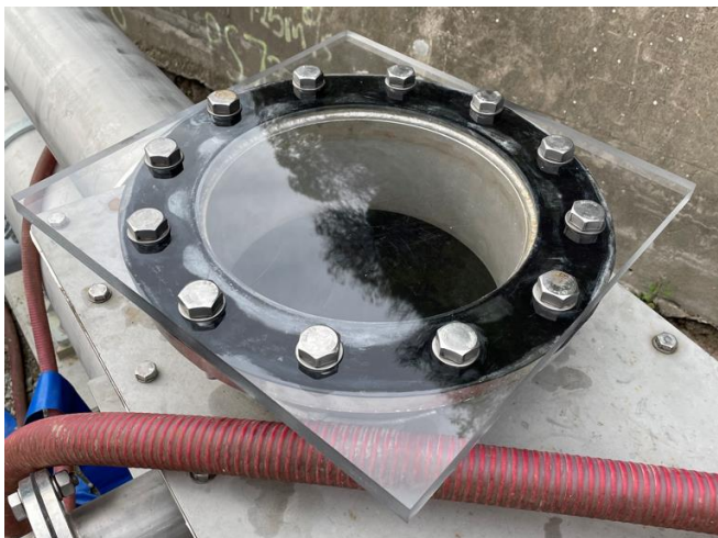
Figure 7: View port installed on the transition chamber
