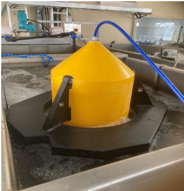
Photo 4: Gas Hood on Aeration Tank
