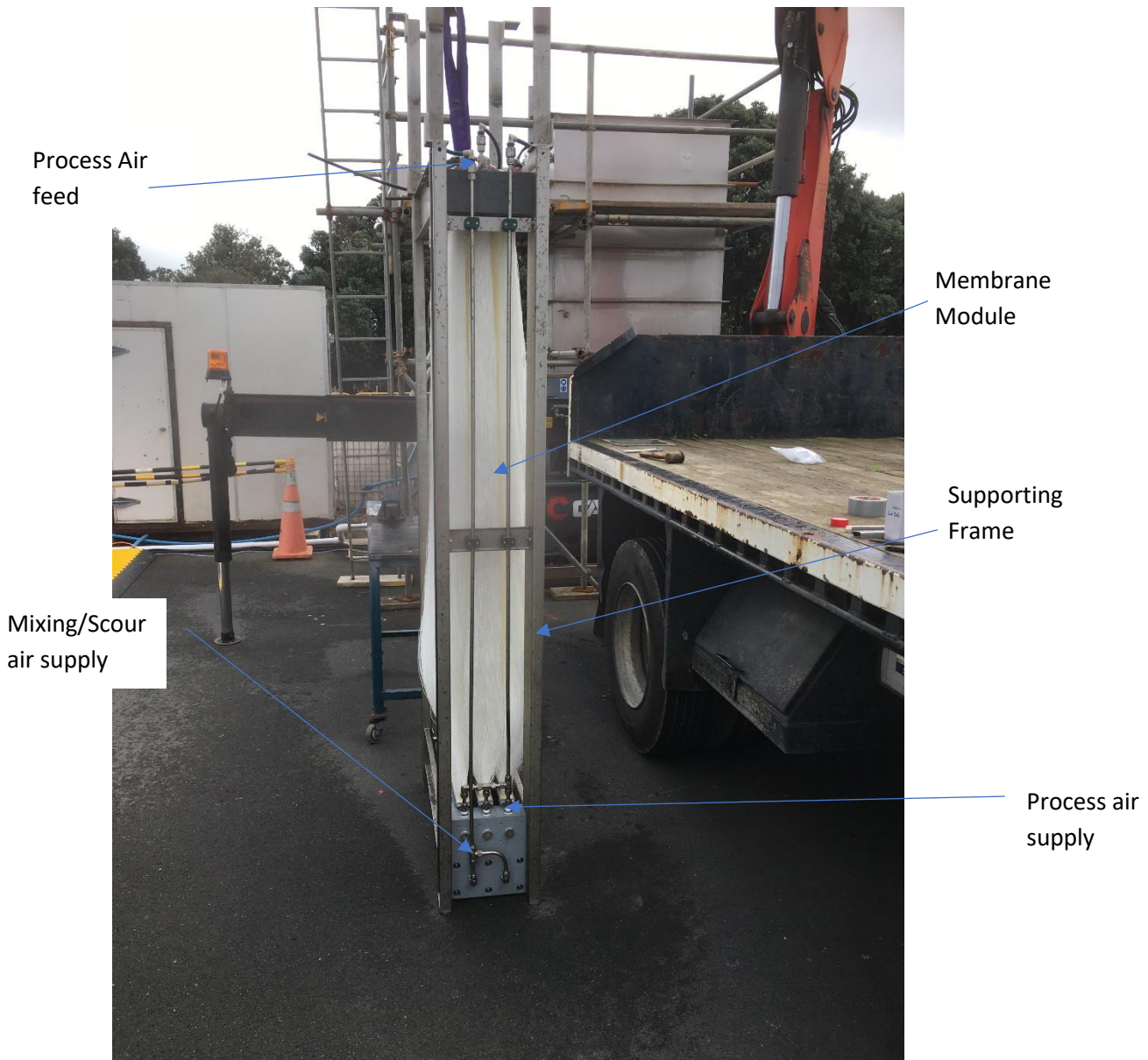
Photo 1: Membrane Modules and Support Frame
