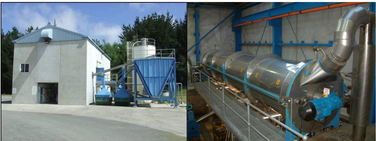
Photographs 1 & 2: Paraparaumu WWTP Sludge Treatment Building (left), and Sludge Dryer (right)
