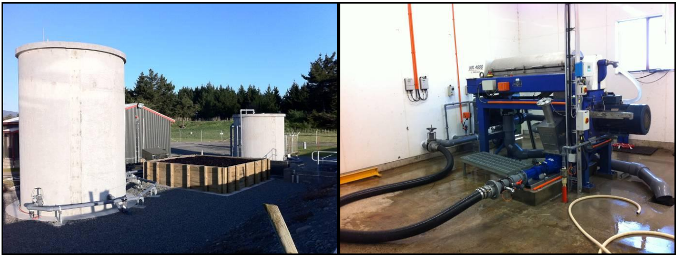
Photographs 3 & 4: Otāki WWTP Sludge Treatment System (left), and Thickening Centrifuge (right)
