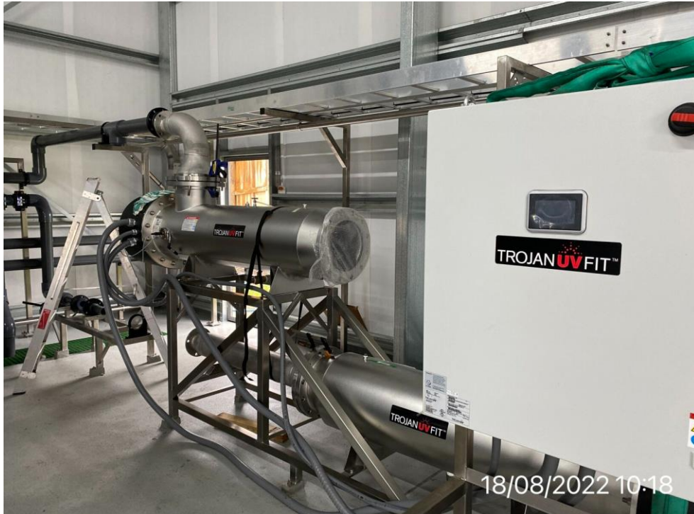
Figure 9: Trojan UV install.
