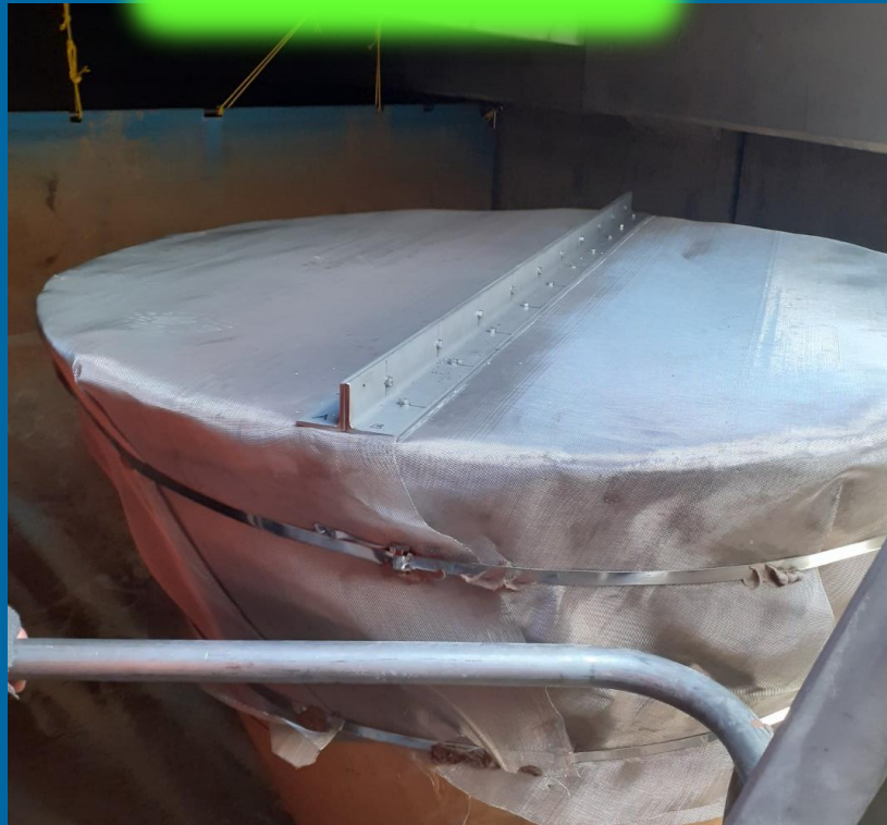
Internal Overflow pipe
