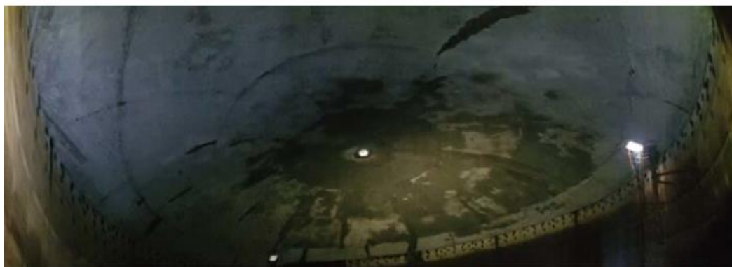
Figure 15: Pre-construction roof leak test, 11 April 2019. Significant dampness around crown and multiple leaks on radial joints.
