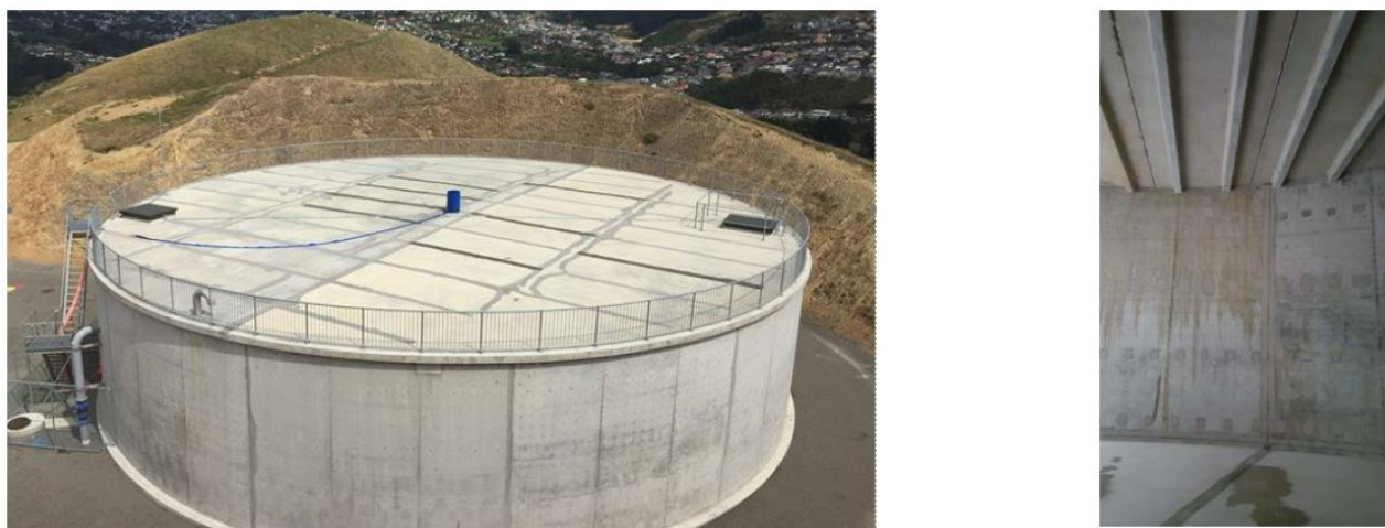
Figure 2 – A new reservoir may score well from a condition rating perspective but may score poorly when subjected to a failure mode assessment due to the roof leakage shown in the photograph on the right.
