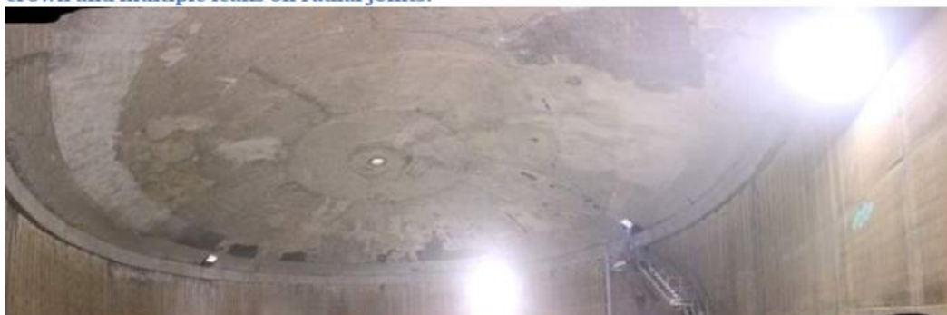
Figure 16: Post-construction roof leak test, 13 November 2019. Note the dark patch repaired areas. Very few (minor only) leaks observed.
