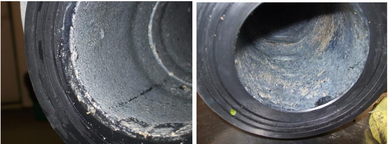
Photograph 4, Photograph 5: Biofilm growth on beginning and end section of 100mm dia. pipe
