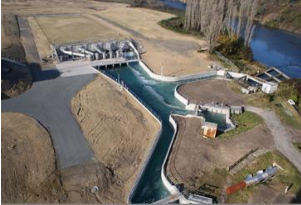
Photograph 9: Completed bioreactor September 2012
