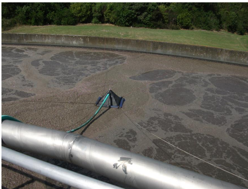
Photograph 6: Gas hood on aeration tank surface
