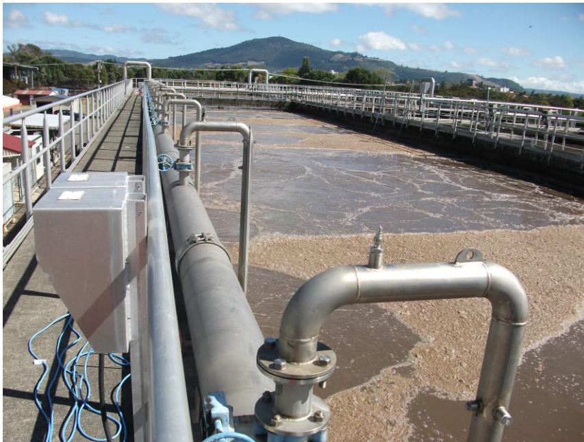
Photograph 5: Dosing nozzles inserted in air dropper
