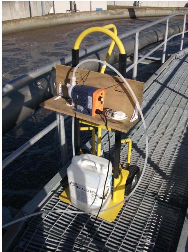
Photograph 4: Dosing equipment (pump on hand trolley and formic acid drum)
