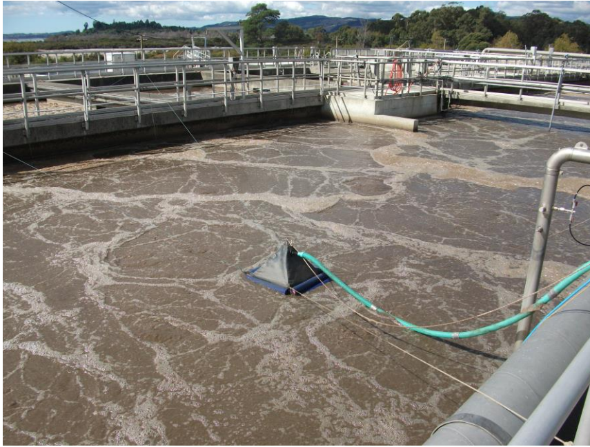
Photograph 3: Gas hood used to collect aeration offgas
