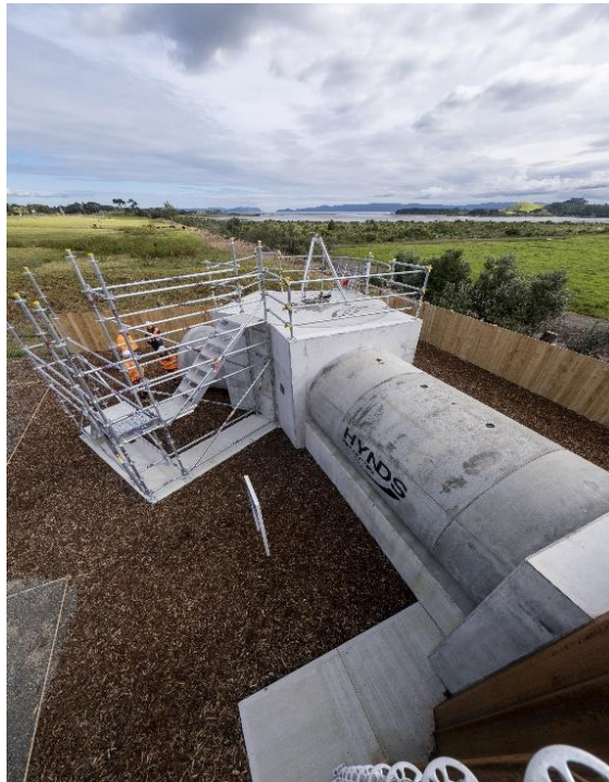
Photograph 2: Raised corbels around the manhole
