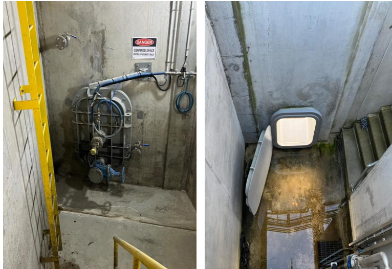
Picture 7 & 8. Access hatches designed into large tanks.
