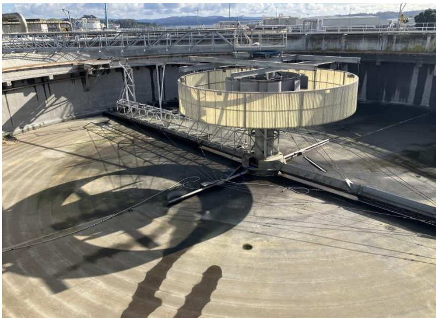
Picture 1. Empty Reactor Clarifier
