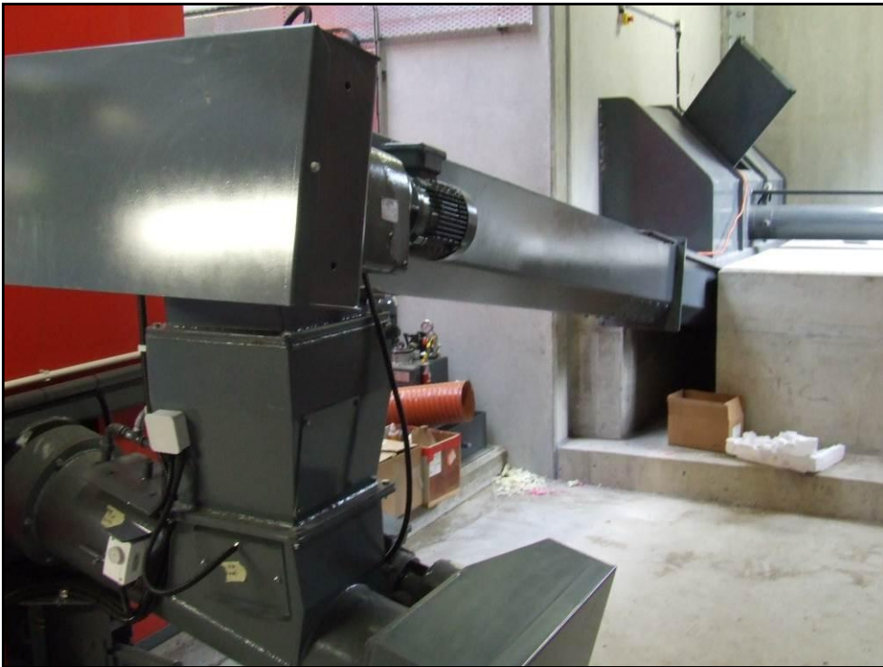
Photograph 5: Fuel Feed System to supply fuel to the New Boiler Unit
