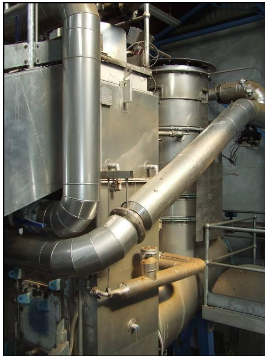
Photograph 1: The Original Diesel Boiler
