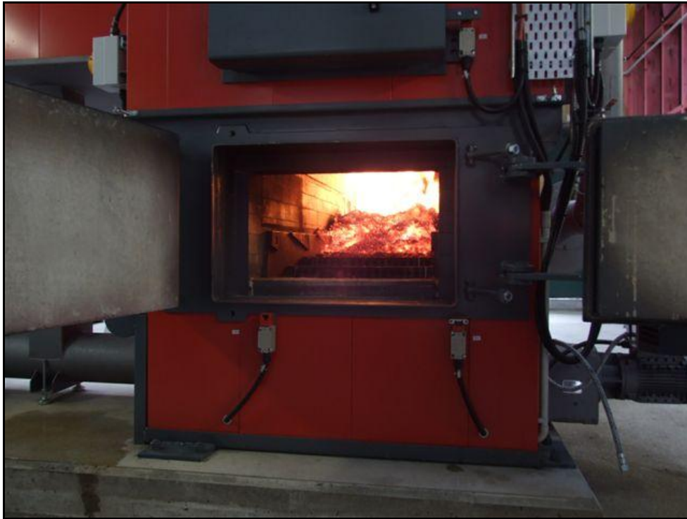
Photograph 8: The Boiler Combustion Chamber in Operation
