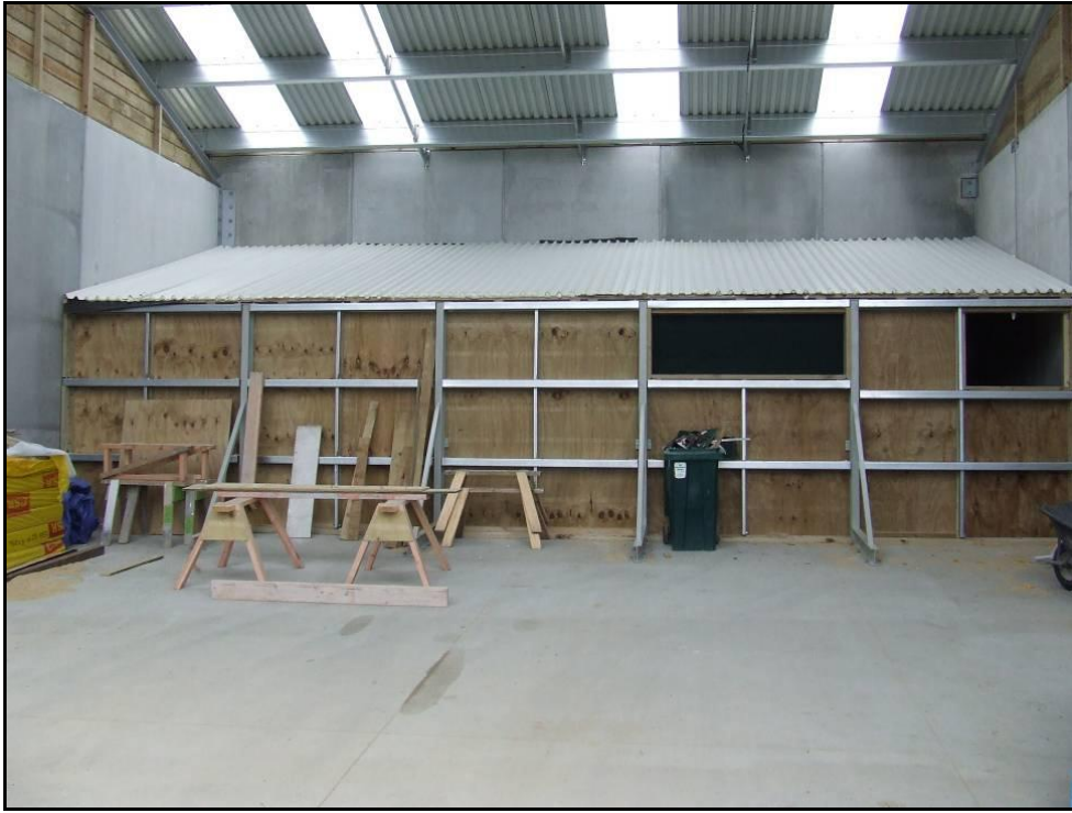
Photograph 4: Containment for Wood Pellets within the New Fuel Store
