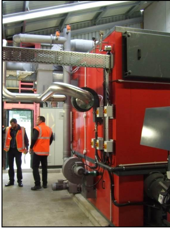
Photograph 6: The New Biomass Boiler Unit
