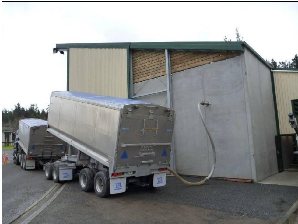
Photograph 7: The First Delivery of Wood Pellets (Pneumatic System)
