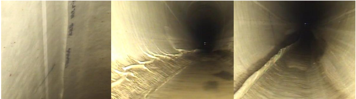
Photograph 2: Example of a minor wrinkle, major wrinkle and a major fin from other CIPP projects
