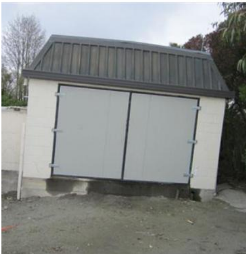
Photograph 1: Rotation of Pump Station 63 resulting from buoyancy uplift, lateral spreading and slope instability
