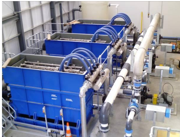
Figure 5: New membrane plant installation at Kerepehi WTP.
