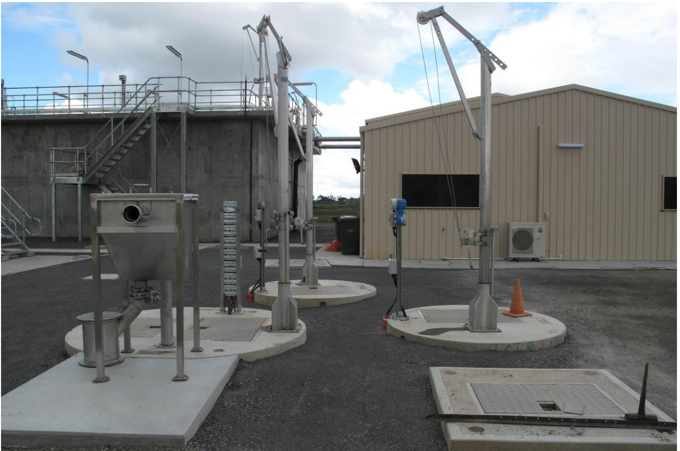
Photograph 10: Septage reception and pumping stations (septage, storm, and transfer)
