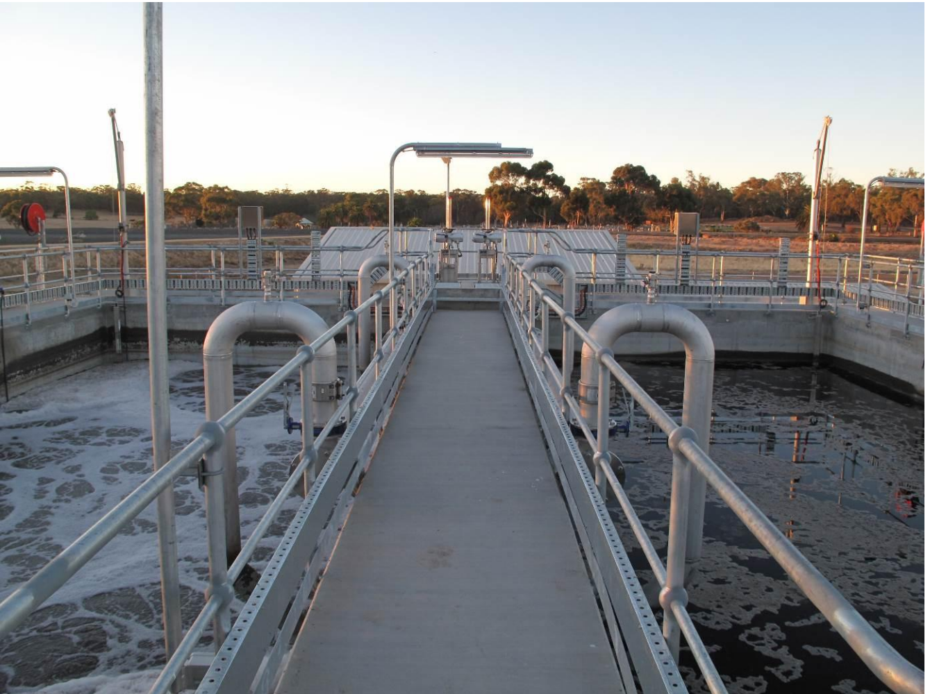
Photograph 6: SBR tanks in operation (aeration phase left, anoxic phase right)
