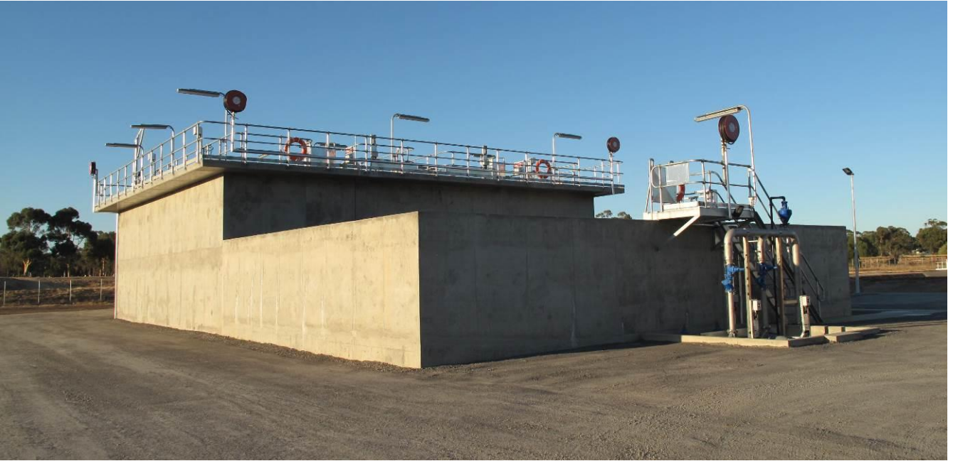
Photograph 7: SBR (taller at rear) and decant tank (foreground)
