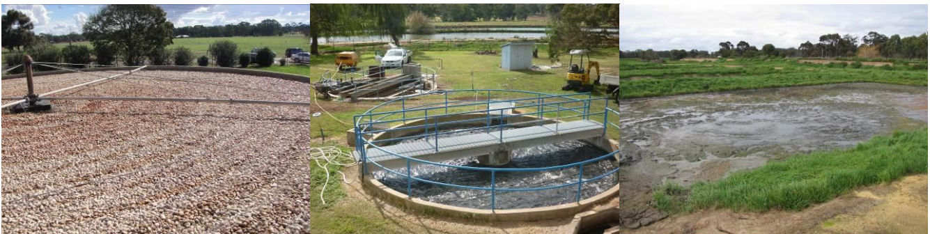
Photograph 1: Old St Arnaud WRP From left to right, trickling filter, Imhoff digesters, sludge lagoon
