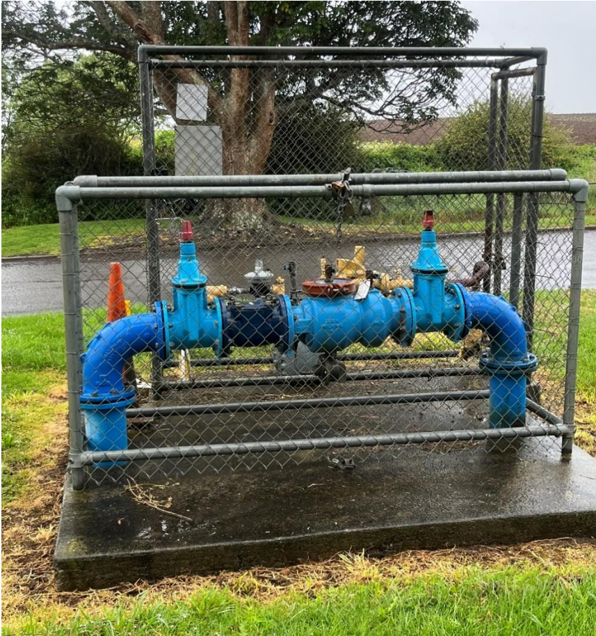
Below: 150mm backflow in a cage - just ok to test, but very difficult to do repairs on.
