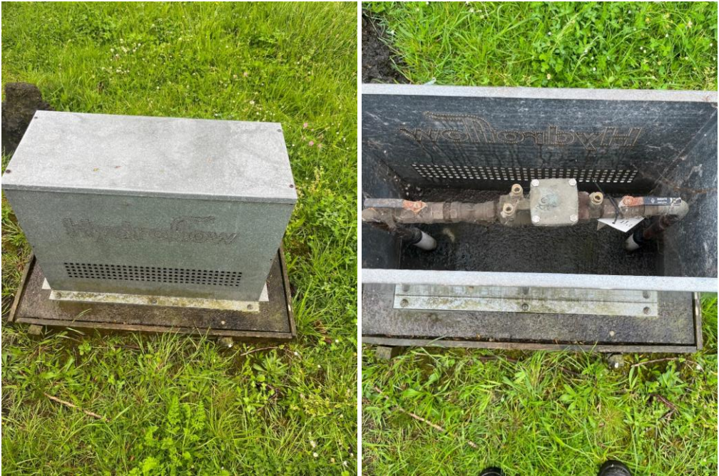
Above: Backflow in a box with screwed lid - easy to remove for testing and repair.
