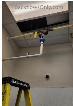
Installed high ... well above the top of the 3m ladder.
