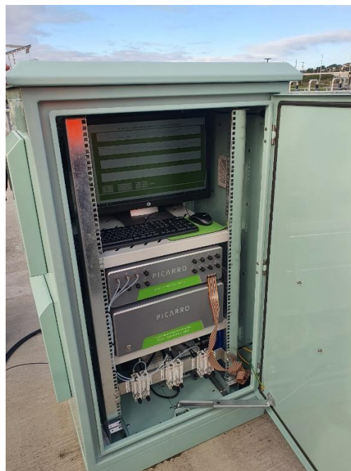
Photograph 2: Picarro off-gas concentration analyser
