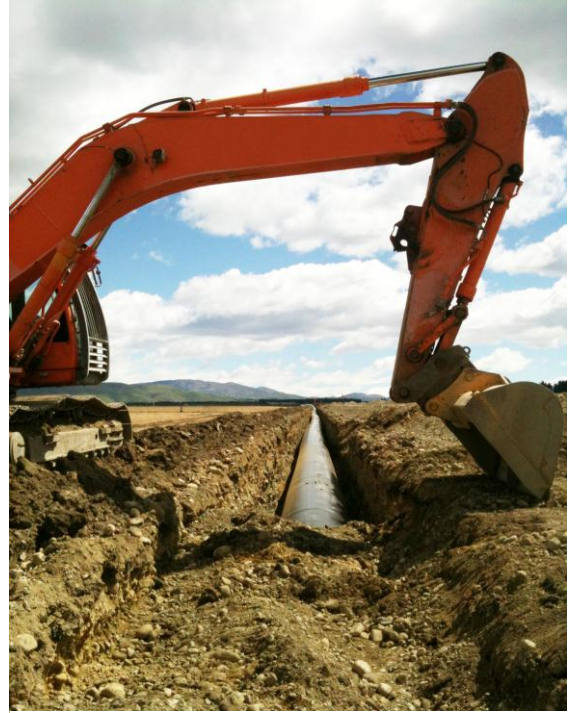
Photograph 3: A typical pipe installation, demonstrating the long straight lengths of pipe that are installed for a piping upgrade
