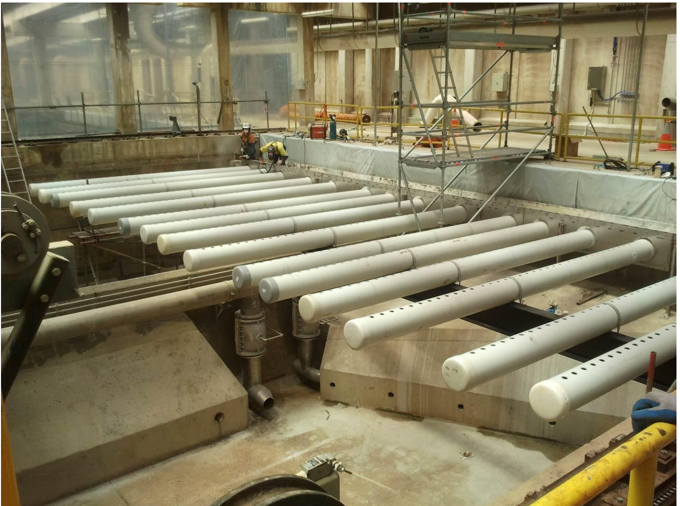
Photograph 3: Outlet end of HRAS tank during construction, showing the submerged outlet launder tubes
