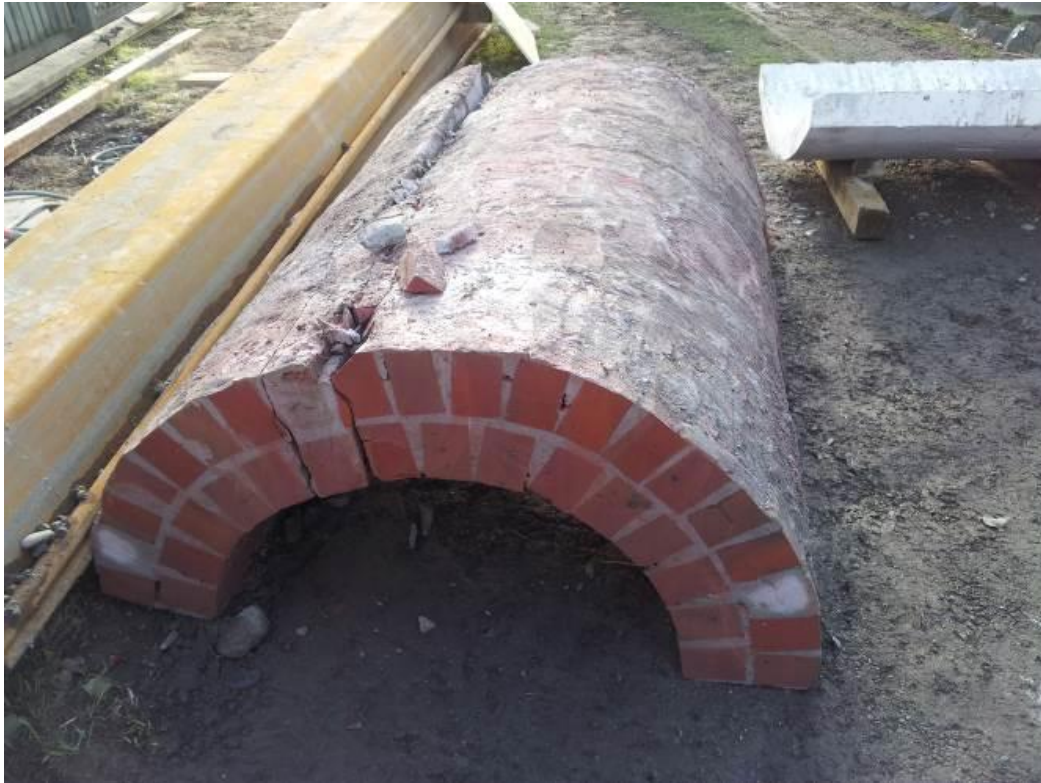
Photograph 11, Section of brick barrel saw cut out and removed intact.
