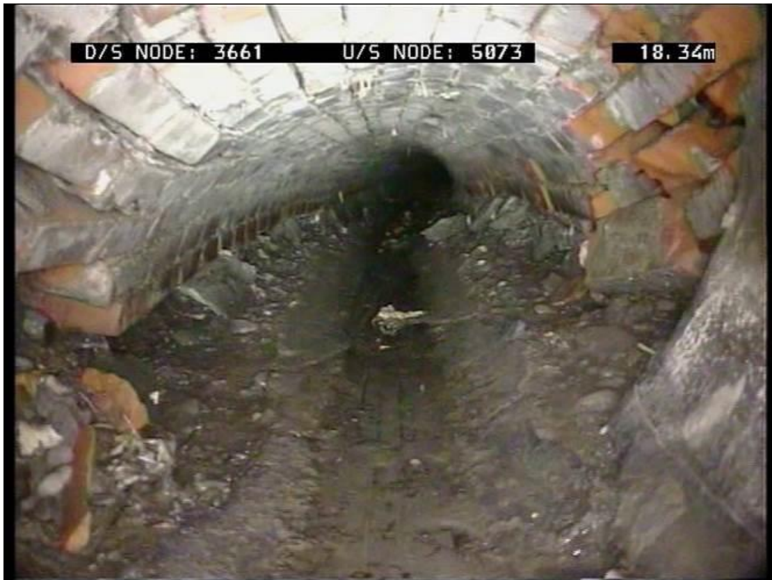
Photograph 1, Close-up CCTV image of 50% collapsed pipe, March 2012
