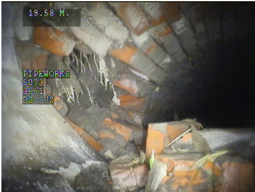
Photograph 10, View of pipe showing hole in wall caused by jet cleaning
