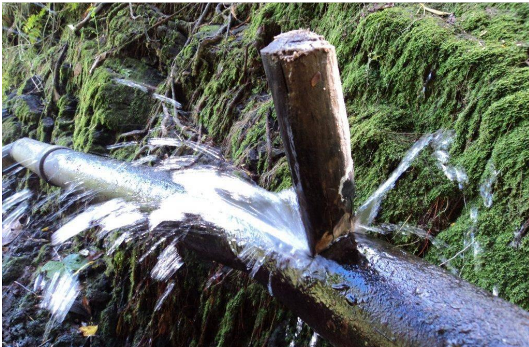
Photograph 9: Air valve – Samoa style.
