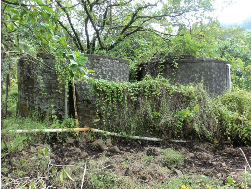
Photograph 8: Existing storage tanks in poor condition.
