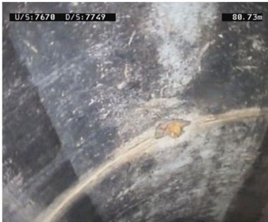
JF-L due to minor concrete damage at joint. IRTS&G requires repair to DN1800 pipe.
