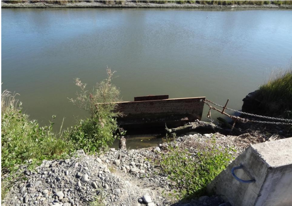
Photograph 2: Steel plate positioned to block a stormwater outlet within the tidal reach of Avon River, New Brighton, to prevent tidal inflow
