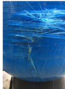
2. Implosion Tank - Broken Fiber Negative Pressure caused by siphon and Pressure Pump (RD) after filtration media tank. No Vacuum Breaker installed. Polyethylene inner shell damaged.
