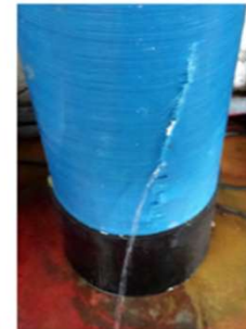
4. Broken Fiber and Inner Polyethylene Shell Negative Pressure caused by siphon and Pressure Pump (RD) after filtration media tank. No Vacuum Breaker installed.
