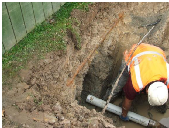
Photograph 4: Restrain™ PVC pipe installed within small confined space beneath existing utilities. Wainuiomata 2012.
