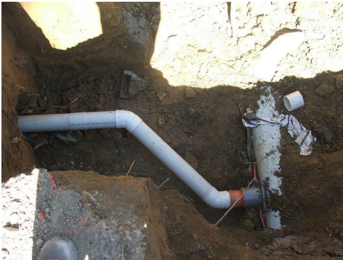
Photograph 9: 3m lengths, DN300 segmented PVC sewer pipes installed by ST-HY-PB. DN100 House Sewer laterals renewed using a ST-HY-PB winch - both pulls employed the CMPTP method. Connections were made using standard SCJ PVC fittings and “Quick Fit Saddles”. Whakatane 2010.
