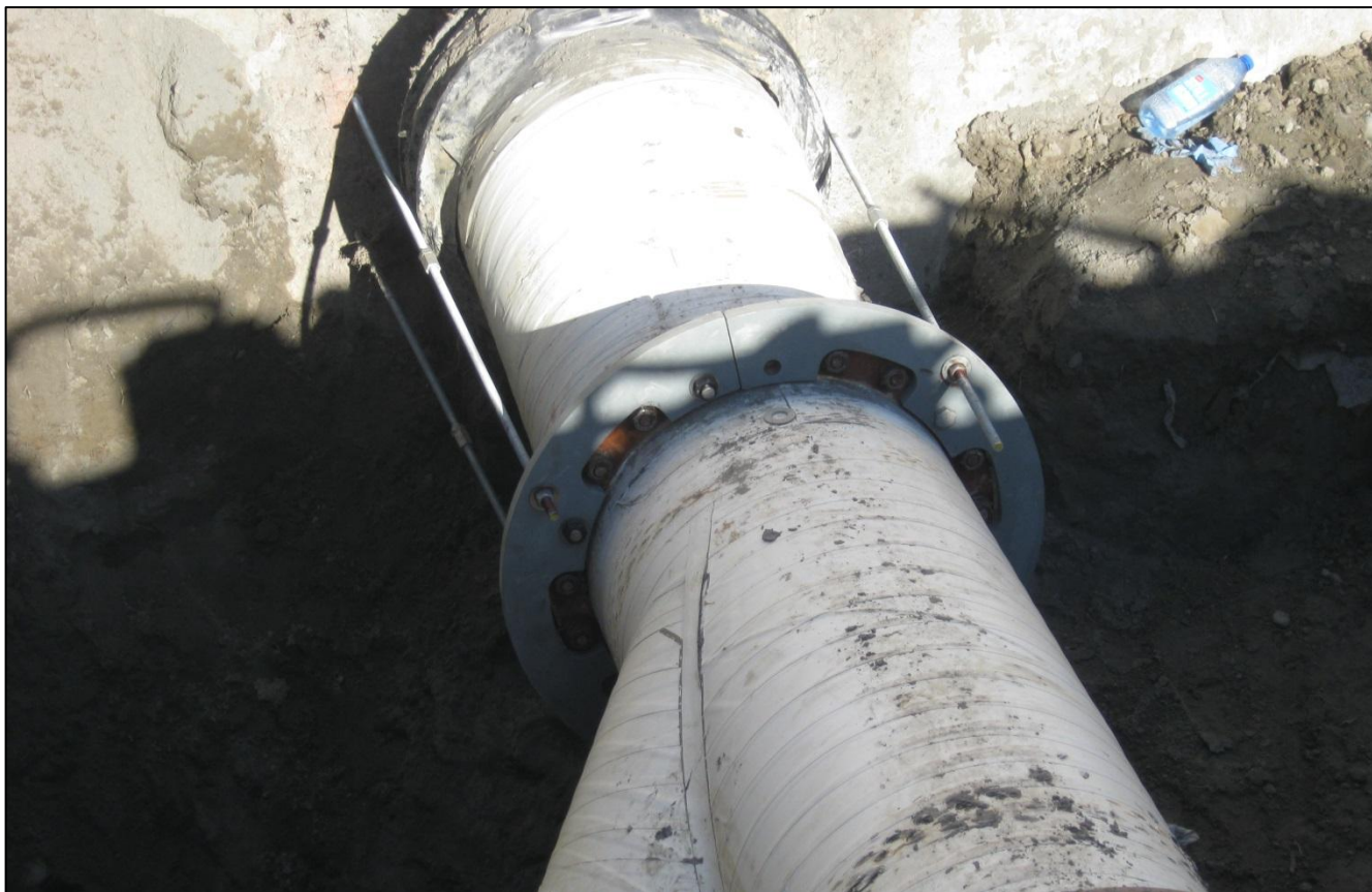
Photograph 10: Post-June 2011 Repairs to Pressure pipe Outlet depicting use of flange modification and steel tie back rods..
