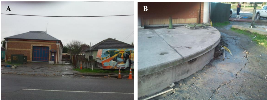
Photograph A: PS36 showing differential settlement and 6° angle of building and wetwell
