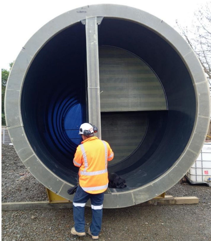
Figure 14: Example of a glass reinforced plastic (GRP) cascade (baffle) drop structure (note "dry side" to the left and the "wet side" on the right)
