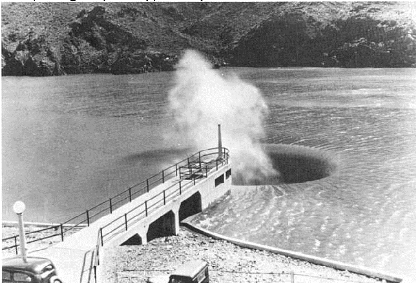
Figure 3: Observed blowback in morning glory drop structure at the Ohywee Dam, Oregon (Falvey, 1980)
