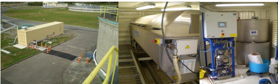
Photograph 4 Photo of Andritz Sludge Booster
