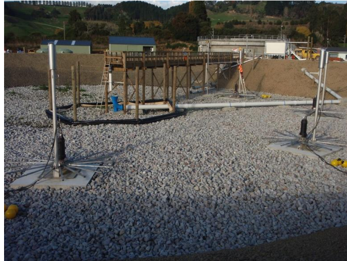
Photograph 9: Floor Mounted Aspirator Aerator
