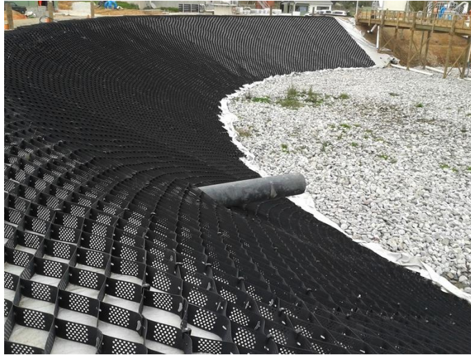
Photograph 2: Unfilled Geoweb Erosion Protection
