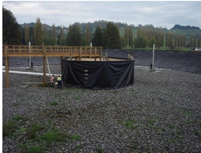
Photograph 5: Curtain Structure for Anaerobic Zone
