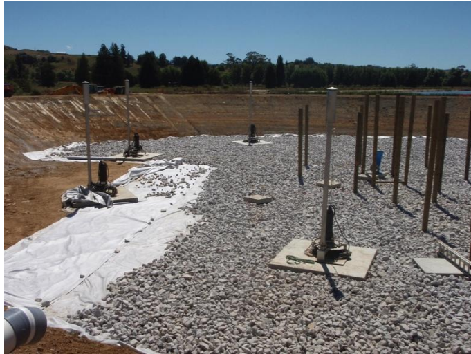
Photograph 1: AS Reactor Earth Bund
