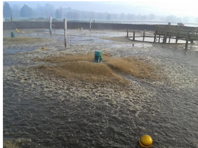
Photograph 11: High Speed Floating Aerator
