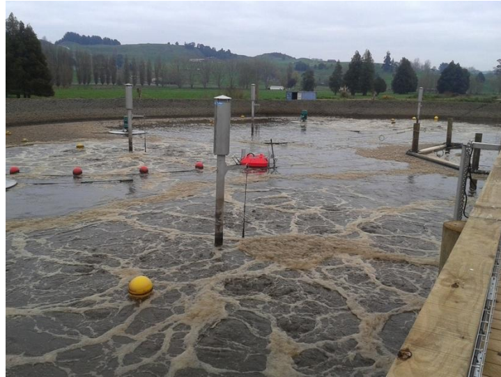
Photograph 10: Floor Mounted Aspirator Aerator in Operation
