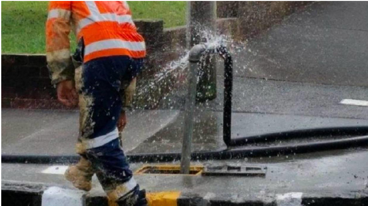
Photograph 2: An offender using an unauthorised standpipe.
