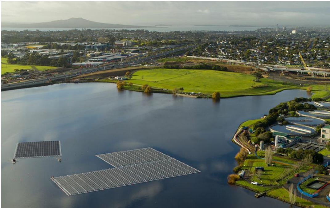
Rosedale WWTP 1,040kW floating array
