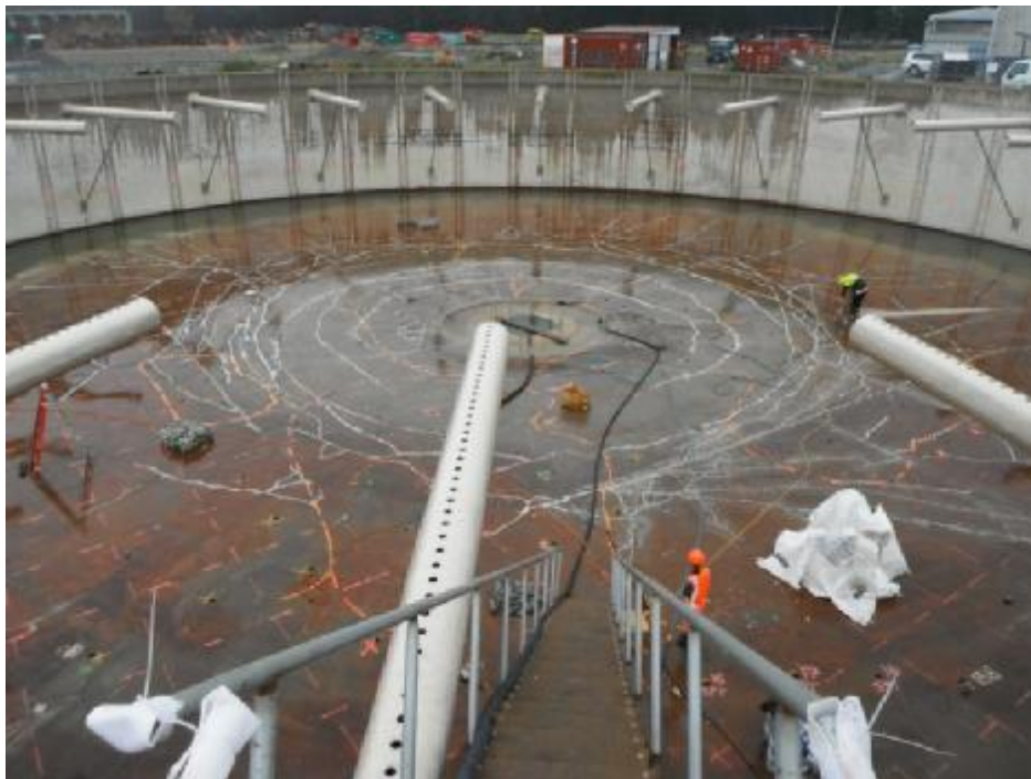
Figure 11: Inverted floor cone on Clarifier 3
