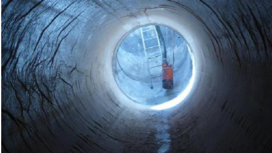
Figure 9: Creasing of Liner on Clarifier 4 Influent Pipe
