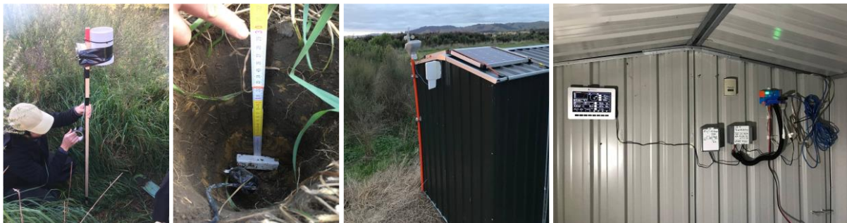
Figure 7: Photos showing, from left to right, the installation of the remote monitoring rain gauge, soil sensor at 30 cm deep, the weather station in the shed powered by solar panels, the interior of the shed with the data receiving and sending devices.
